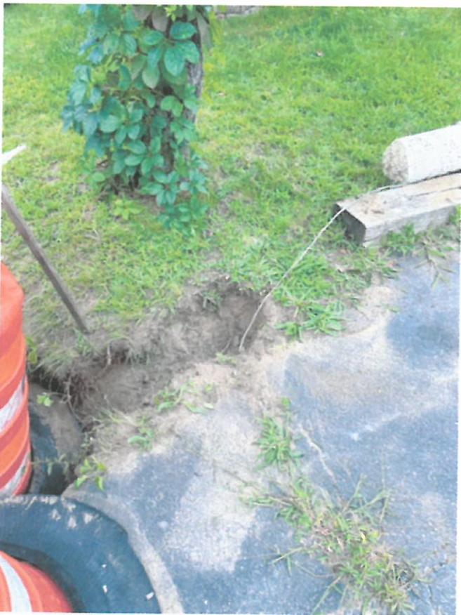
The electrical wire is 2' away from the hole and runs under and across the driveway to the light with burned out electrical
