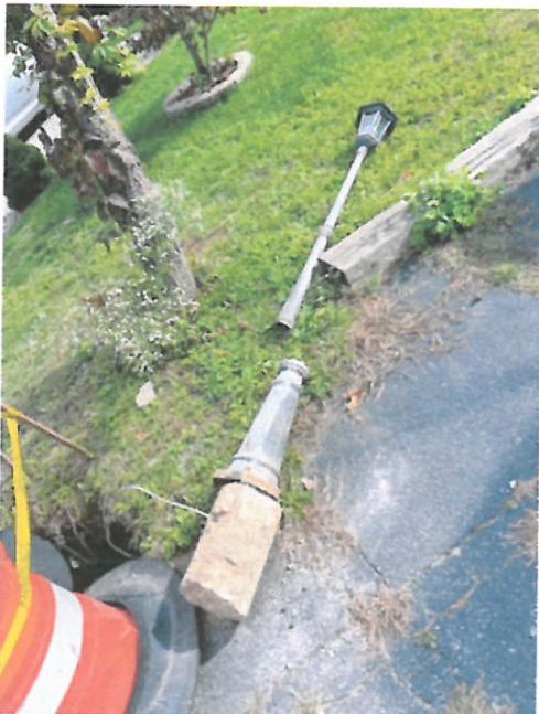
Light pole & broken base
