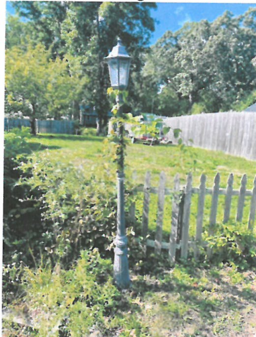
Light on opposite side of driveway electrical and wiring burned out.
