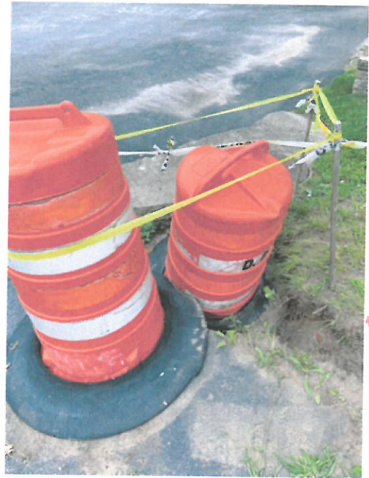
The orange can & pad covers the washed away part of the driveway
