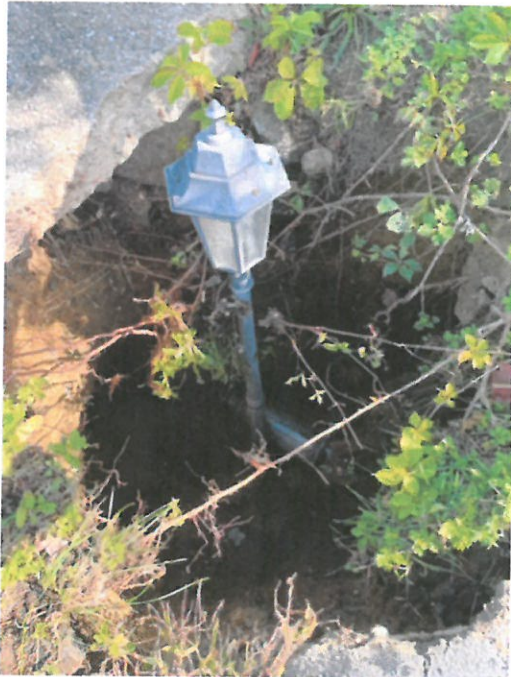
Broken light & light base swallowed by the 7' hole.
