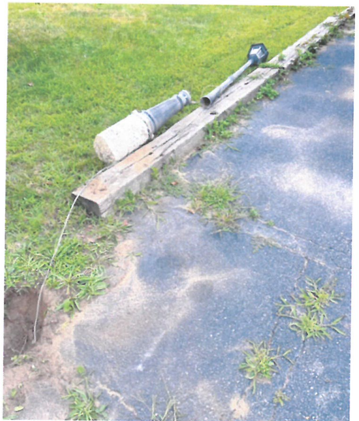
The broken light base and light pole are now well away from the hole.
