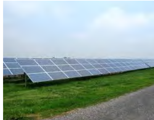
Figure 3: Sample Installed Solar Array Note: proposed site will be mounted on ballast blocks rather than embedded posts.
