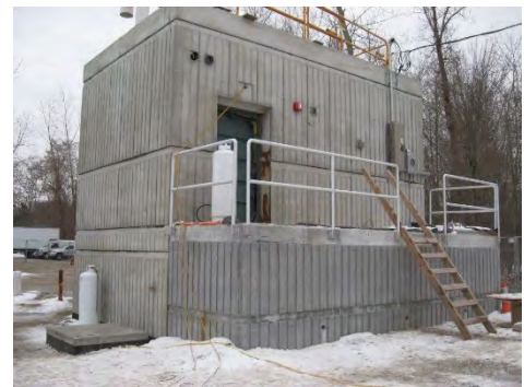
Elevated Bellows Street pump station protected from 500-year floods (2017).
