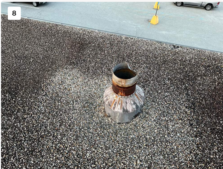
Damaged roof top equipment
