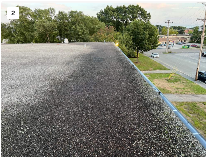
Ponding conditions along the perimeter
