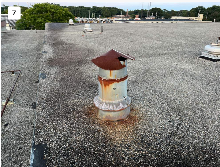
Damaged roof top equipment
