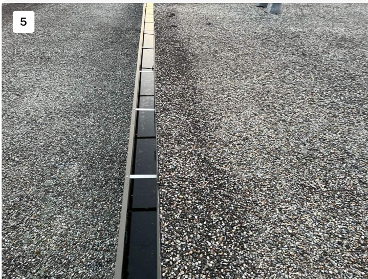
Clogged gutters - typical
