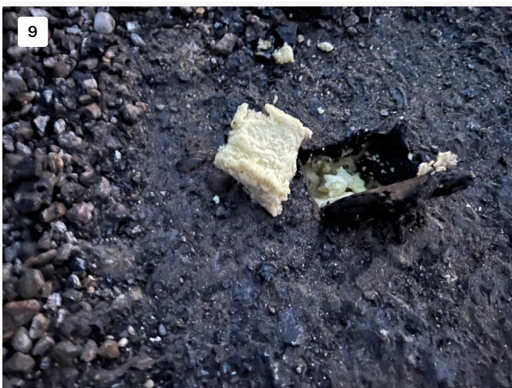
Wet insulation @ Test Cut #6
