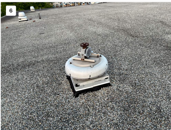
Damaged roof top equipment
