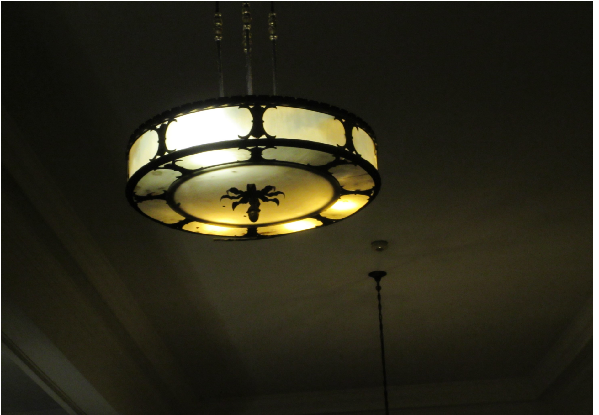
Detail of light fixture, Auditorium, Aldrich Junior High School
