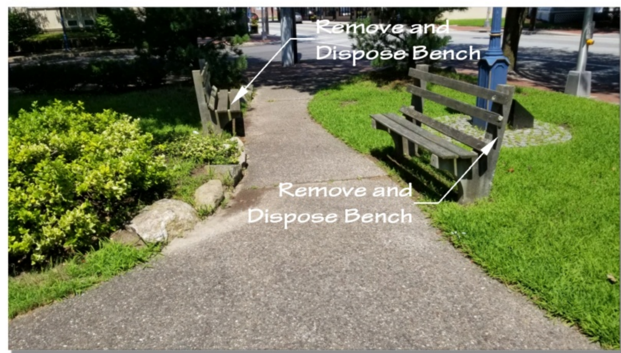
E Donovan Park - West Shore Rd. entry. Remove and dispose of two (2) existing benches and footings. Install 10' W X 3' L X 4" thick concrete pad. Install surface mount Dumor #58 black steel bench or approved equal.
