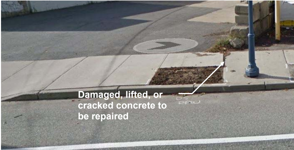
Figure 6 – Example of sidewalk area to be repaired. Remove existing panel, install compacted processed gravel as required, install wire mesh reinforcement and fill pit with 4" of 3000 PSI rated concrete. Finish to match surrounding walkway.
