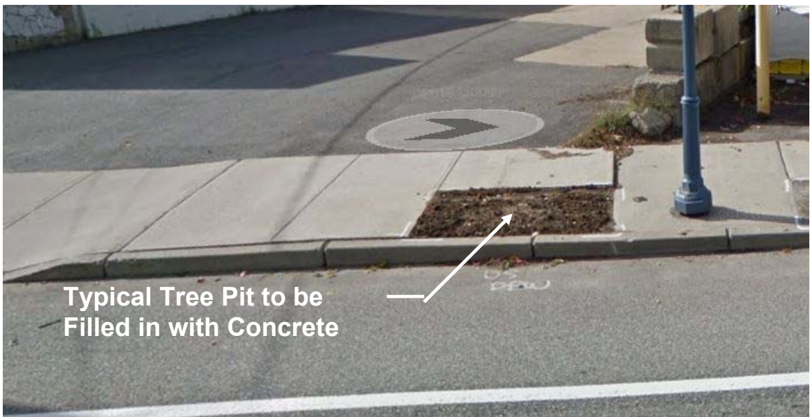
Figure 5 – Typical tree pit to be filled in. Excavate 10" below finished sidewalk grade, install compacted processed gravel, install wire mesh reinforcement and fill pit with 4" of 3000 PSI rated concrete. Finish to match surrounding walkway.
