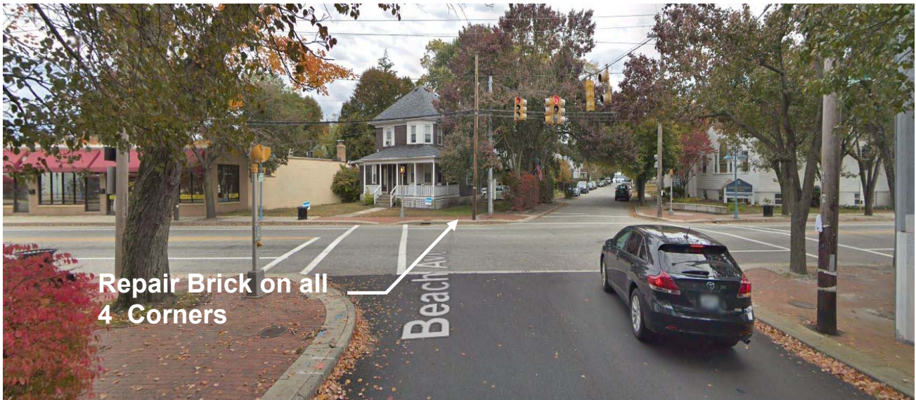
Figure 9 – Brick work located within the right of way at the intersection of Beach Street and West Shore Road shall be power washed and cleaned. After brick is cleaned install new polymeric sand as outlined in Section 32 14 16.
