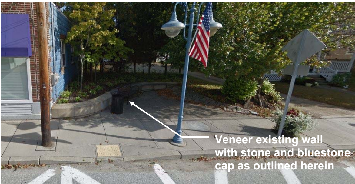
Figure 13 –Existing wall adjacent to 801 West Shore Road. Veneer wall with natural thin stone with bluestone cap as outlined in Section 04 41 00.
