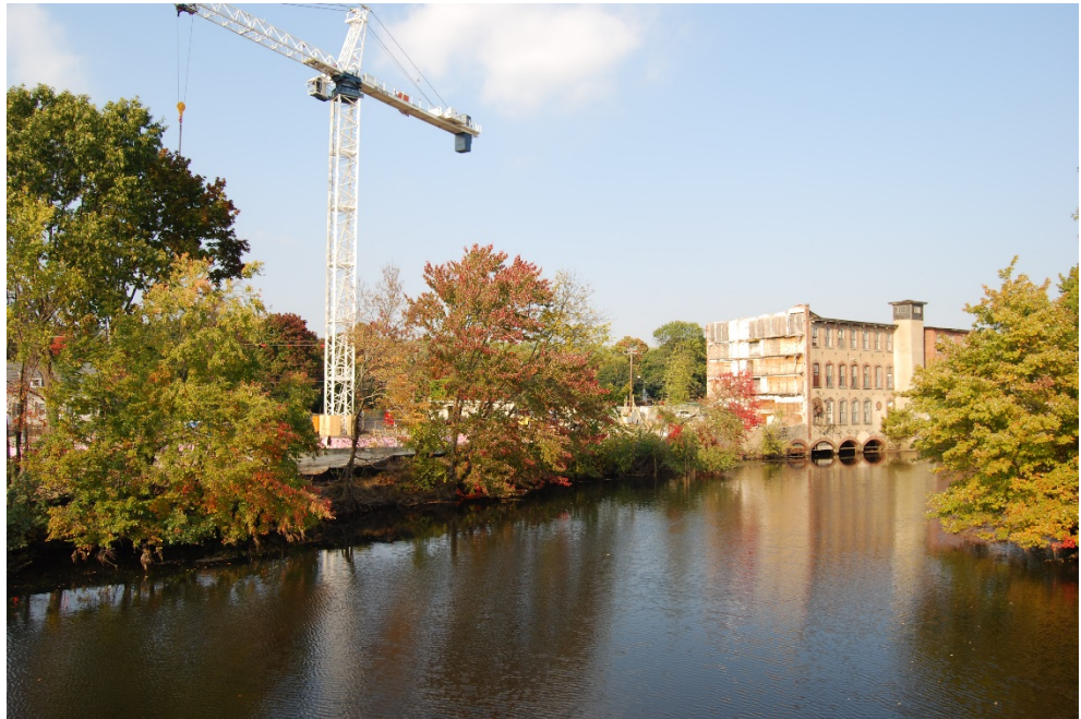
Reconstruction of Pontiac Mills (Nylo Hotel) along the Pawtuxet River after the 2010 Floods.
